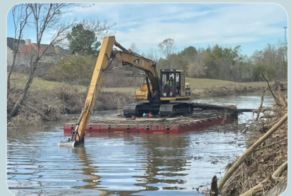
The photo above shows dredging of Ward Creek Source: Amite River Basin Drainage & Water Conservation District
